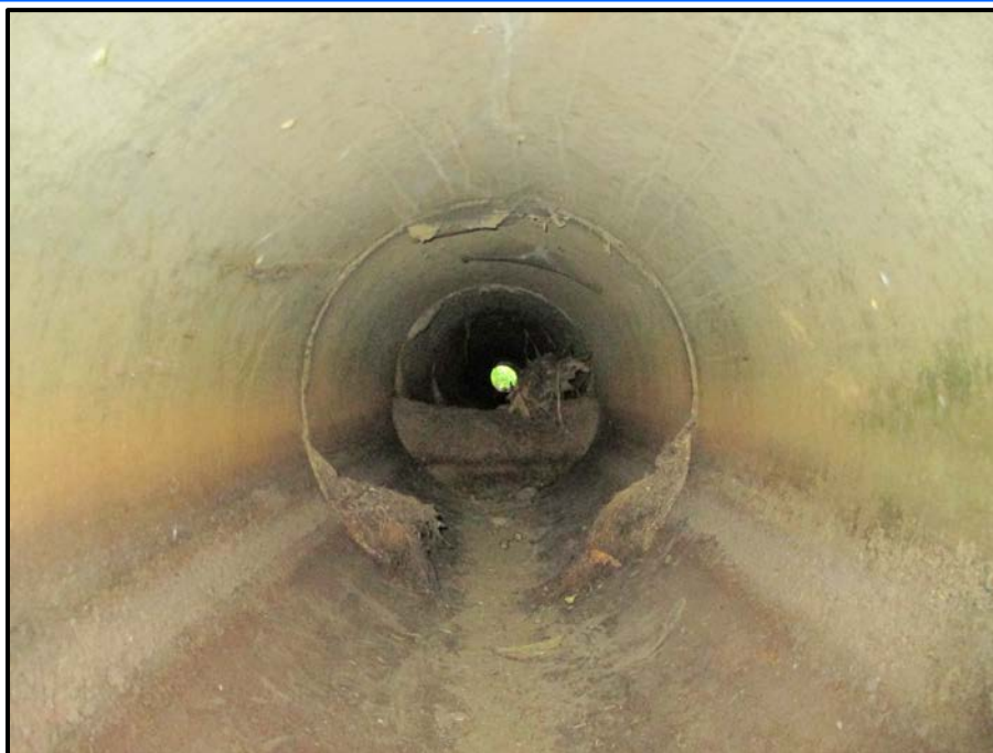
Photo Number: 3 General underside view looking west (upstream), south pipe. Note tree root growth. Photo Taken: 09/15/2016
