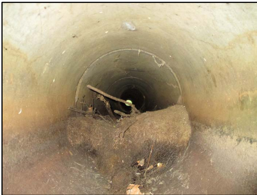
Photo Number: 4 General underside view looking west (upstream), north pipe. Note tree root growth. Photo Taken: 09/15/2016
