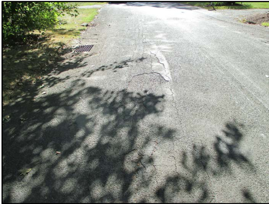
Photo Number: 7 Widespread cracking, settlement, and developing potholes Photo Taken: 09/15/2016 throughout the northbound lane.
